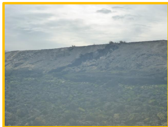
Significant voiding along north face of North Gare Breakwater (/C0503C01)
