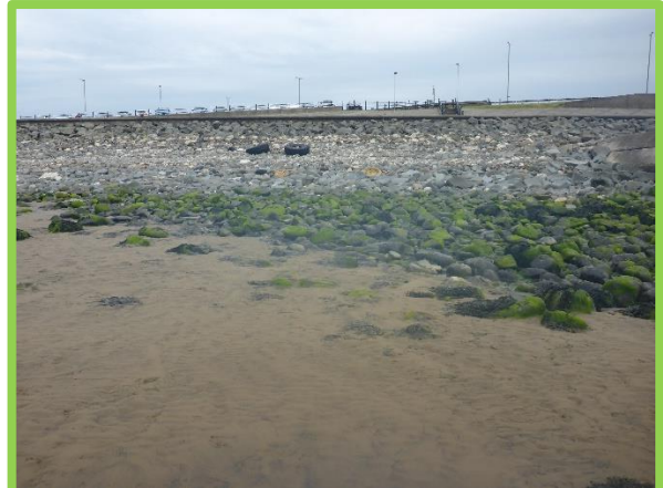
Displaced rock at toe north of Newburn Bridge outfall structure. (/C0401C33)
