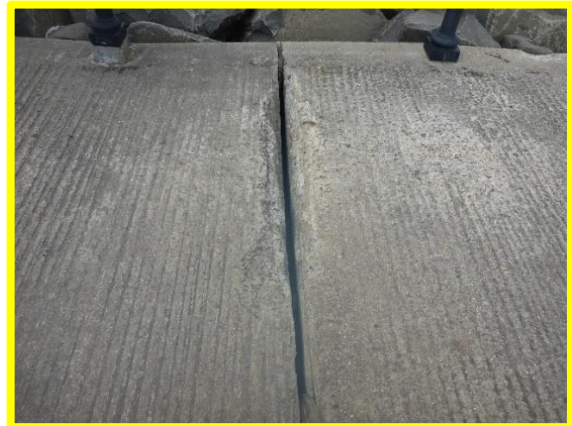
Loss of flexible joint sealant in northern access ramp (/C0401C33)
