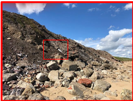
Exposed pipework in made ground slope (C0302C02)
