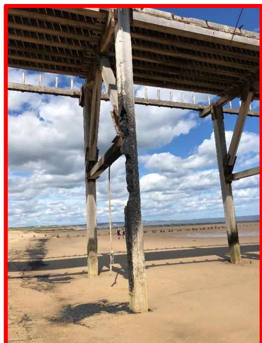
Loss of section to pier support columns, likely due to fire damage (/C0302C01)
