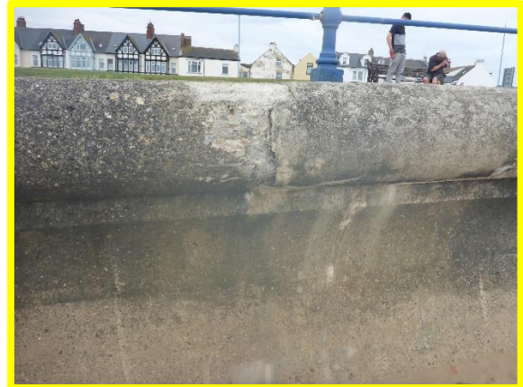
Defect in concrete cope. (/C0501C05)
