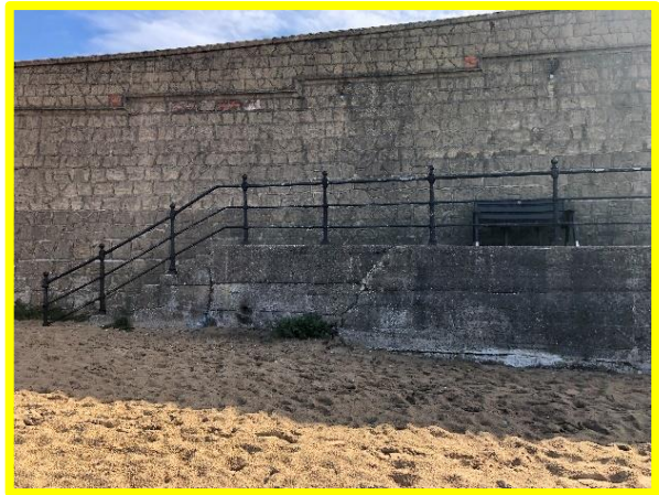
Cracking to access steps (/C0401C35)
