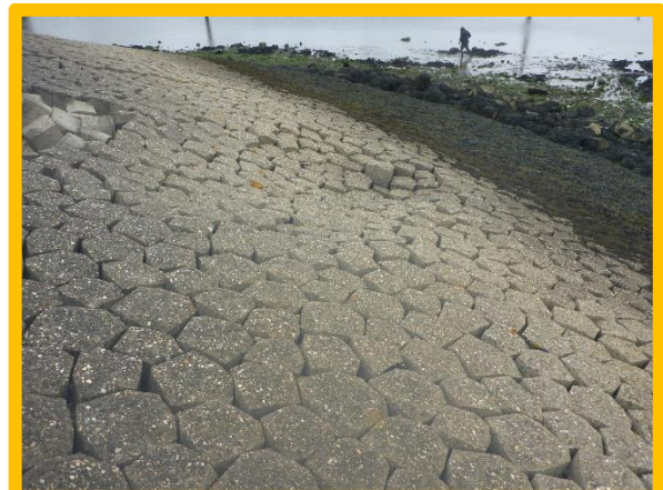
Local settlement of concrete blocks not worsened since 2018 (C0401C26)
