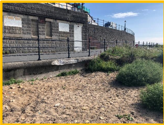
Damaged cope and cracking to former public conveniences (/C0401C05)
