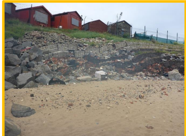
Stacked gabion wall in poor condition especially to the south. (/C0401C17)
