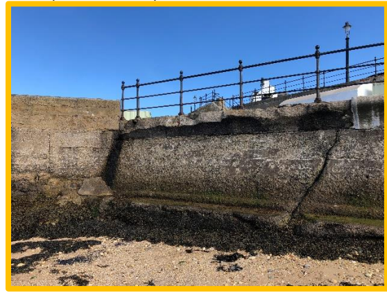
Spalling damage to recurve wall, significant crack suggesting settlement. Old Pier to left of image (/C0401C05)
