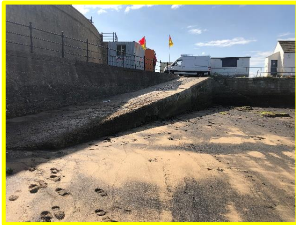
concrete repair to slipway hidden by shadow, voids/undercutting remains (/C0401C35)
