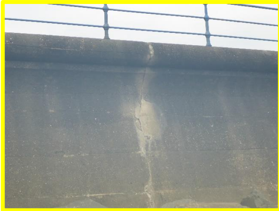
Local cracking and spalling of concrete (/C0501C05)
