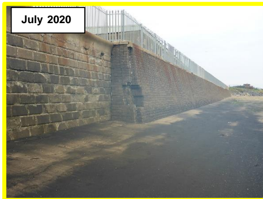
Loss of blocks doubled in size since 2018. High beach levels concealing scour. (/C0401C19)
