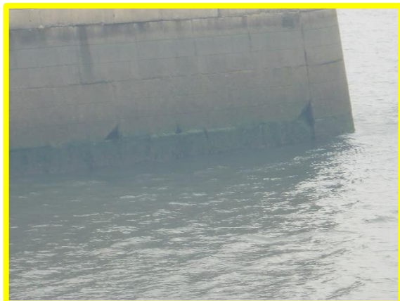
Voids in pier head of North Pier (C0401C22)
