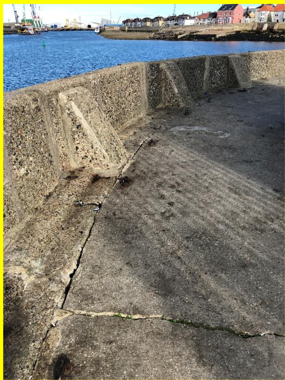
Cracking in parapet wall and deck (/C0401C34)
