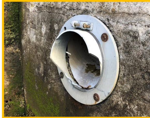
Broken Flap Valve (/C0401C04)
