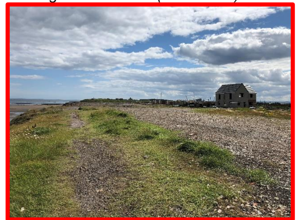
Property development on former industrial site, fronted by collapsed gabion structure (C0302C02)
