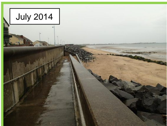
Exposed rock armour berm at Little Scar access ramp (/C0401C33)
