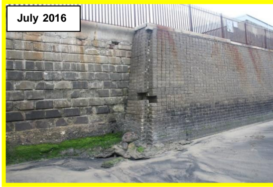
Missing blocks at interface between two walls. Local scour at toe (2016) (/C0401C19)
