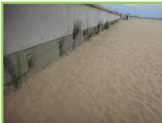
Vegetation growing in joints – should be removed (/C0501C04)
