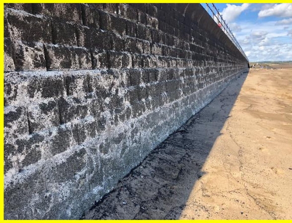
Abrasion to lower levels of seawall (/C0303C01)
