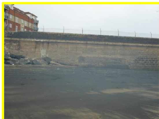
Vertical crack through parapet and seawall /C0401C20
