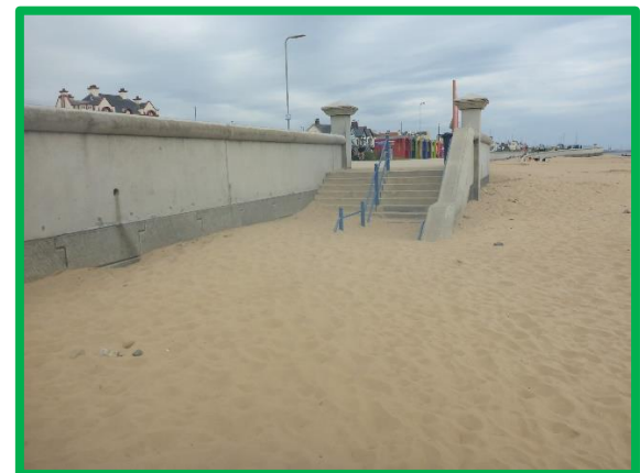
High beach levels at access steps (/C0501C04)
