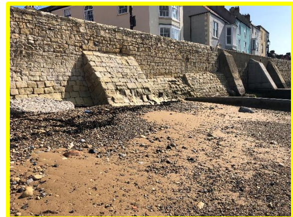
Open jointing in lower masonry courses and heavily abraded masonry blocks (/C0401C35)
