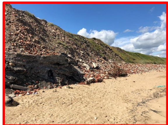
Erosion of made ground slope and collapsed former gabion structure (C0302C02)
