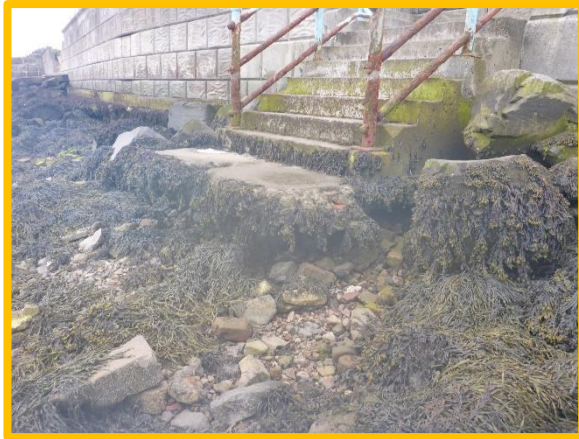
Undercutting of access steps (/C0401C27)
