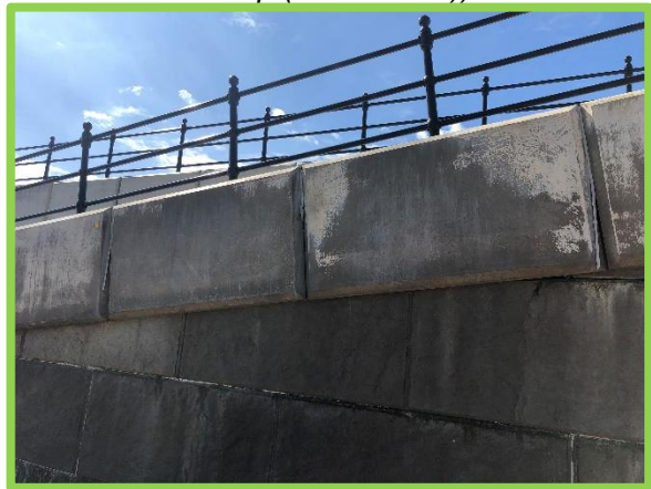
Sealant being washed out of newly installed cope stones (/C0303C01)
