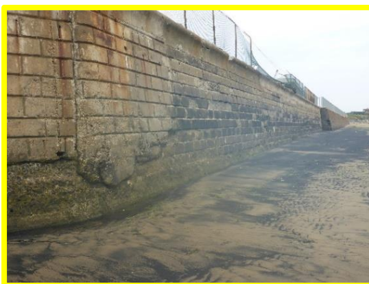
Spalling/abrasion of concrete blocks (/C0401C19)
