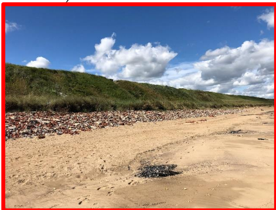
Burst brick gabions spread along foreshore to the north (C0302C02)
