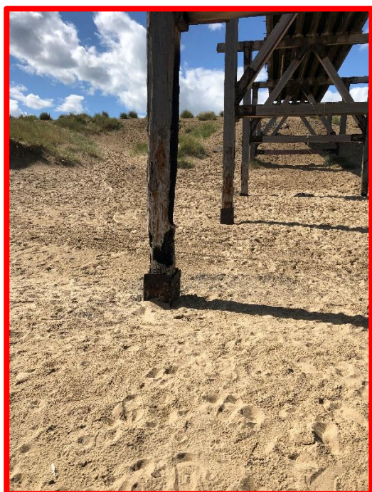
Loss of section to timber support columns of historic pier structure, likely due to fire damage (/C0302C01)
