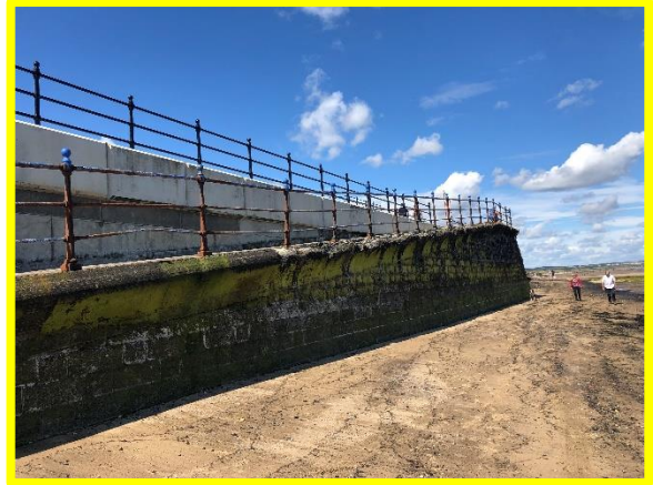
Local damage to coping/handrails at Thorpe Street access ramp (/C0303C01)
