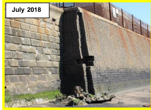
Progressive loss of blocks at interface between two walls. Local scour at toe (2018) (/C0401C19)
