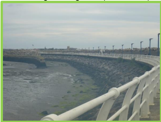
Inner face of South Pier. Vegetation can be seen on crest. (/C0401C32)
