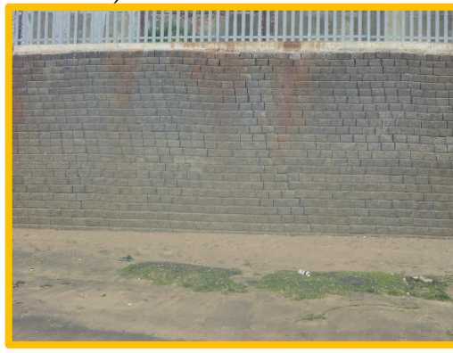
Inconsistent profile, missing copes, open joints (/C0401C19)
