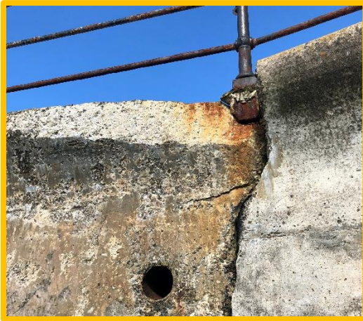
Damaged cope around handrailing fixing (/C0401C04)
