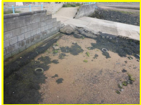
Low beach levels exposing undercutting of concrete toe to the west. (/C0401C27)
