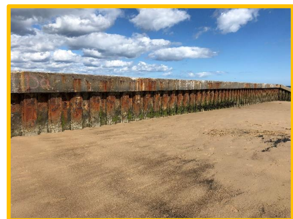
Heavily corroded piled outfall structure (/C0302C01)
