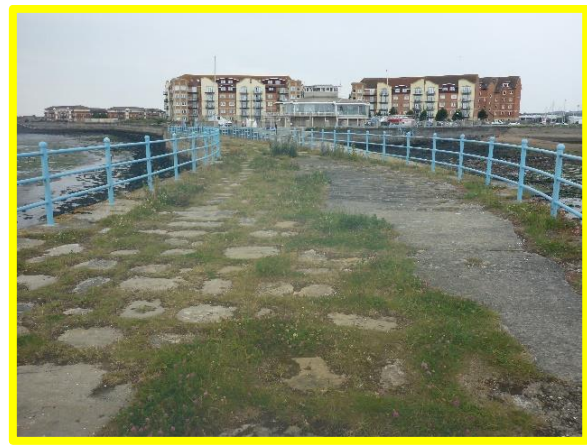
Extensive vegetation growth through joints in Middle Pier deck (/C0401C28)
