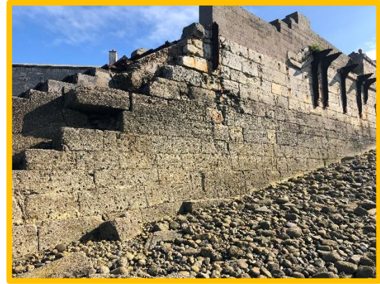
Damage to steps at former passenger ferry landing (/C0401C35)
